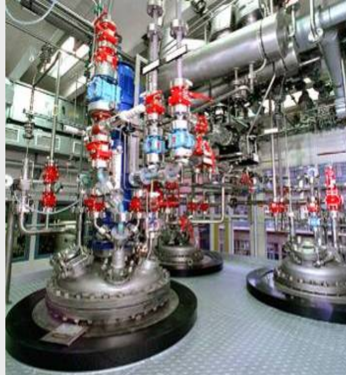
400 I reactors and distillate receivers
